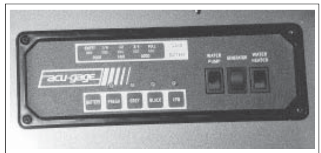
Fig. 12-13 WATER HEATER SWITCH
