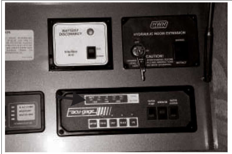
Fig. 10-13 BATTERY CONDITION METER
