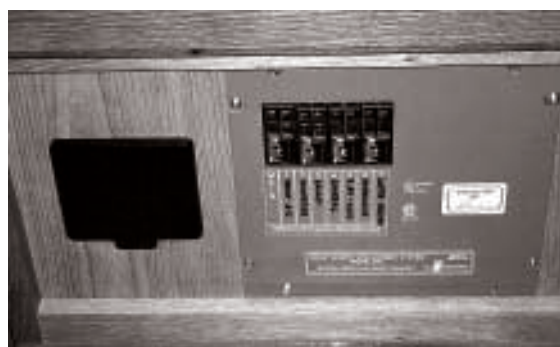
30 Amp EMS Breaker Panel
