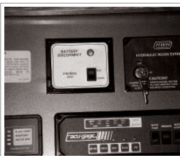
Fig. 10-10 AUXILIARY BATTERY DISCONNECT (COMMANDER ONLY)
